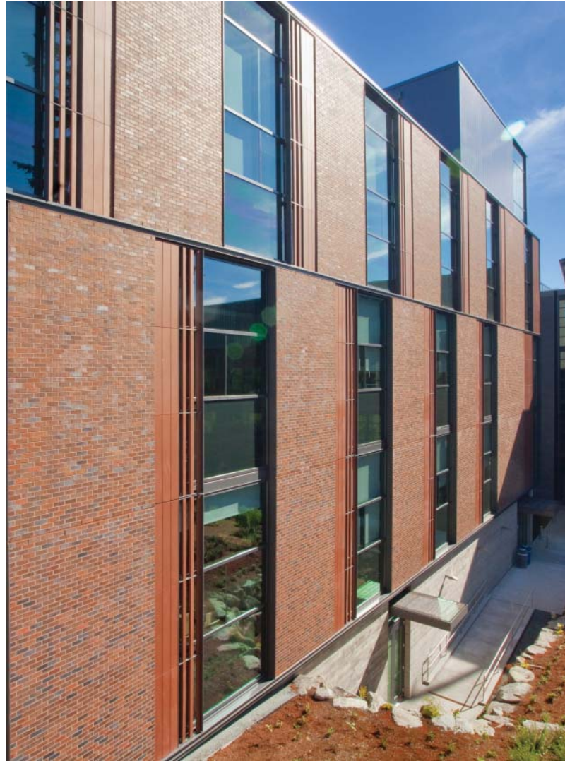
Thermafiber® RainBarrier® 45 continuous insulation (ci) was installed on the University of Washington Bothell, Discovery Hall in Bothell, WA.
